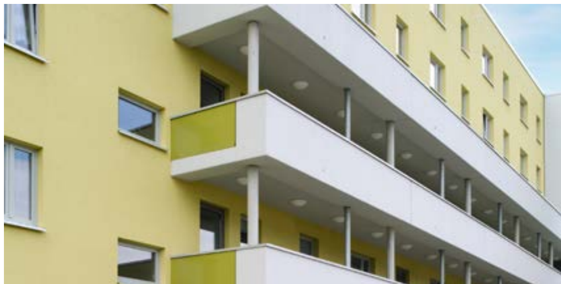
Multiple dwelling, Greifswald, DE StoCretec expertise: StoFloor Balcony Elastic EB 200, strengthening structures with Sto S&P CFK plates Photo: Maximilian Meisse, Berlin
